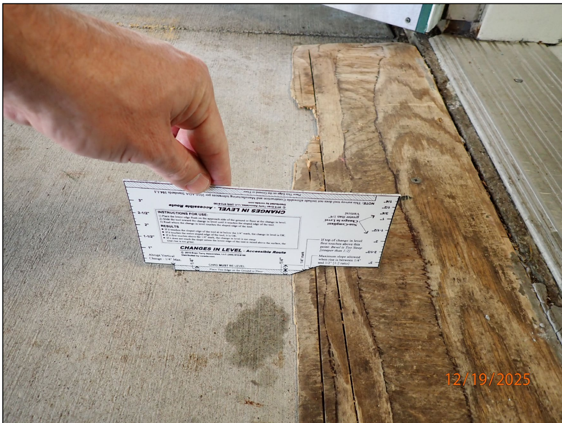
Item 9 – Some retrofitted thresholds have worn and require replacement.
