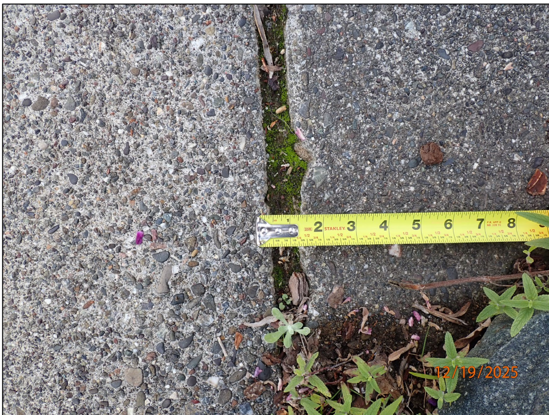
Item 4 – Gaps greater than 1/2” at site flatwork.
