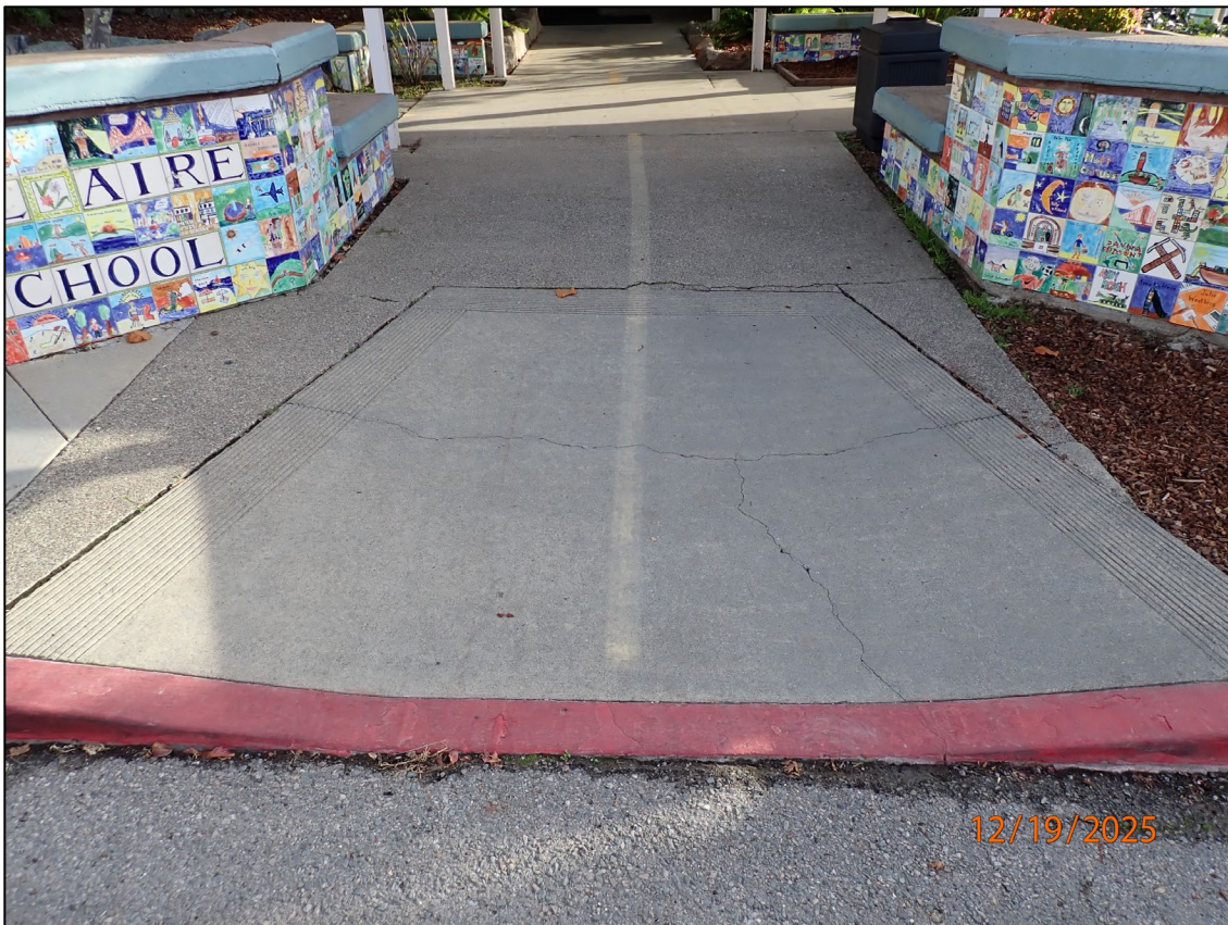
Item 2 – No detectable warning at curb cut.
