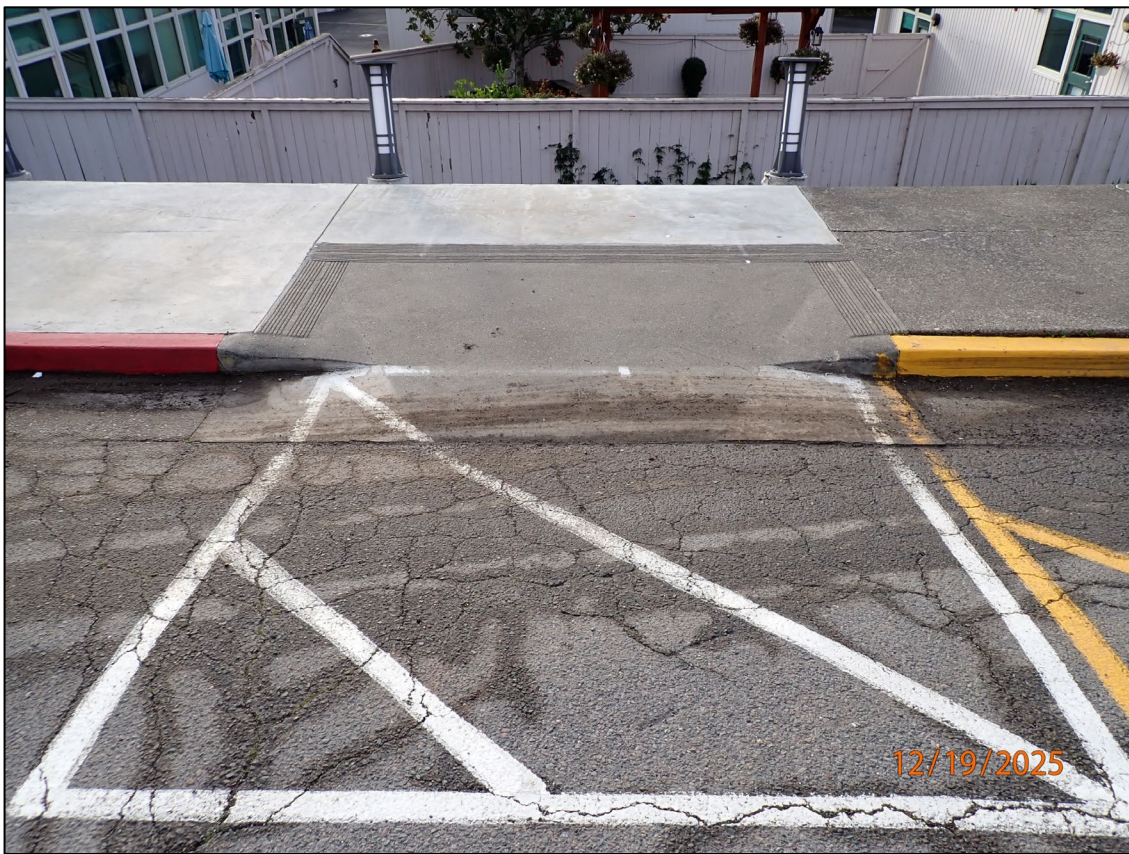
Item 2 – No detectable warning at curb cut.
