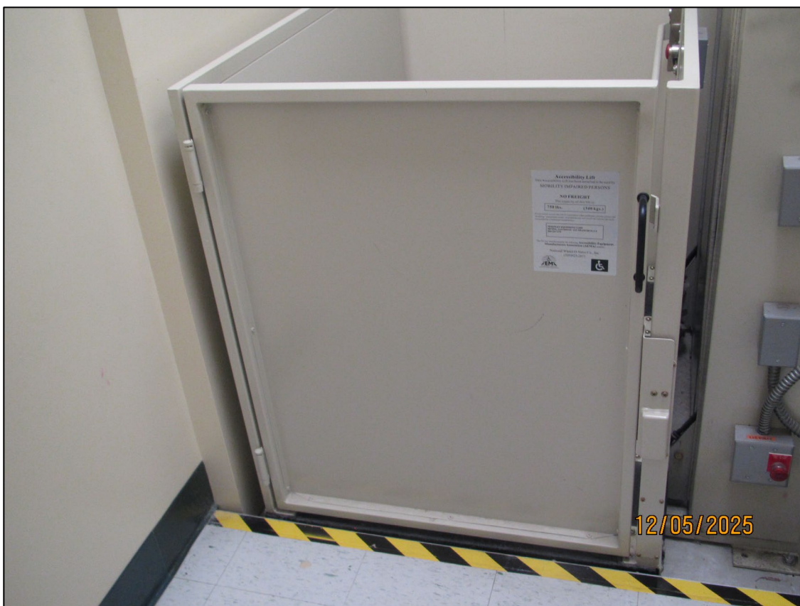
Item 8 – Lift installed in multipurpose room to provide stage access.
