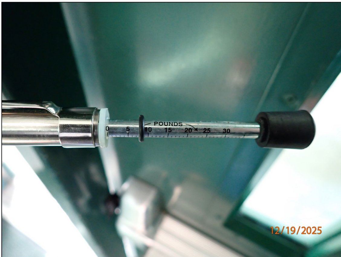
Item 3 - Door operation requires greater than 5 lbs. pressure.
