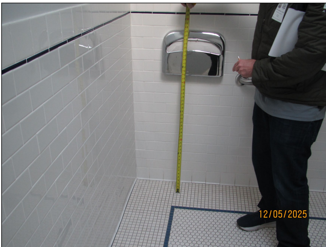
Item 13 – Toilet seat dispensers have been installed within reach range.
