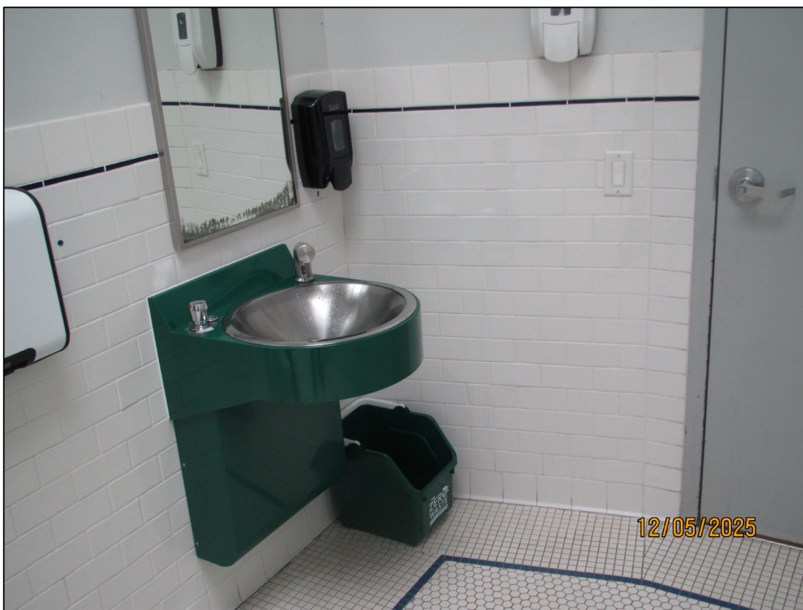
Item 15 – Sinks have knee and toe clearance and cover plumbing components.
