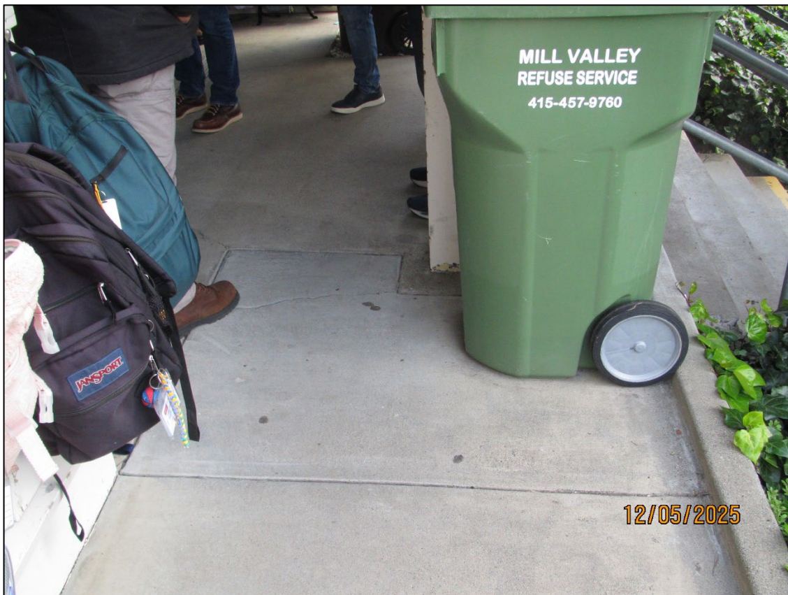
Item 5 – Trash cans obstruct the accessible route.
