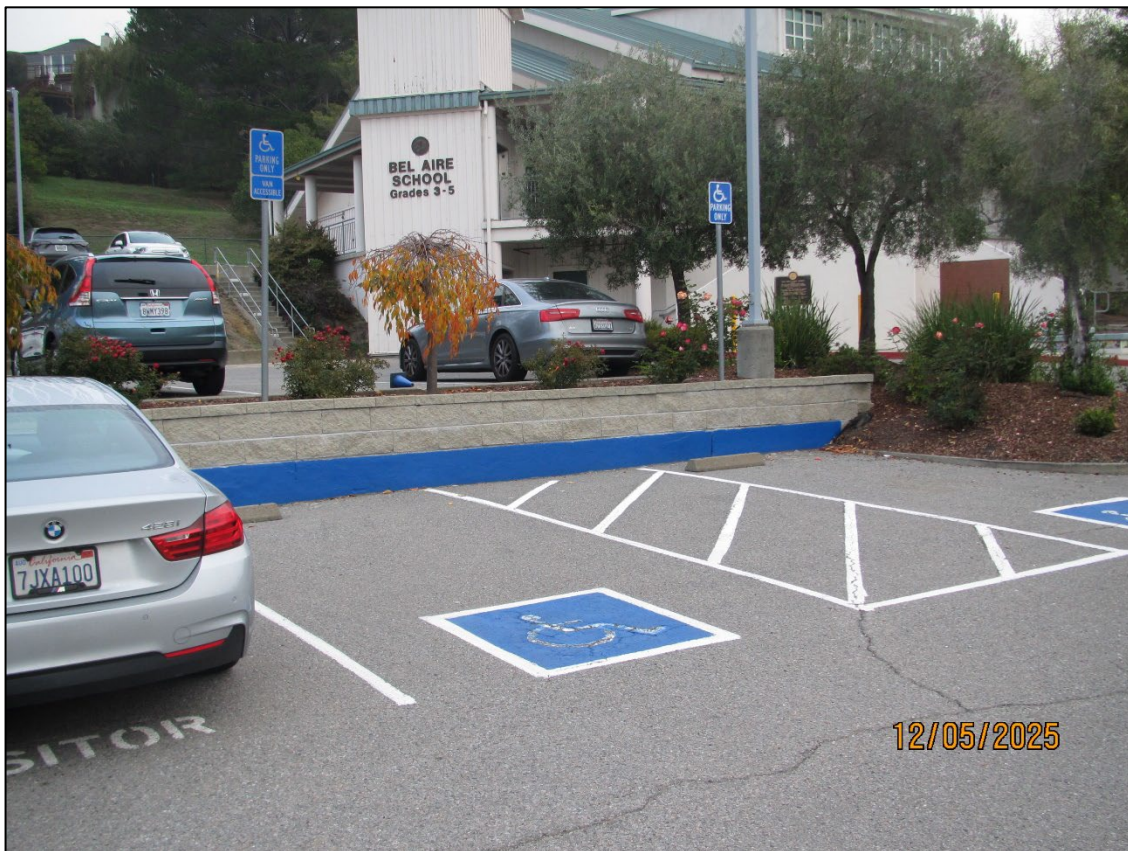
Item 1 – Accessible parking spaces. Minimum fine signs are absent.
